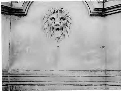
Figure 28: Evidence of inappropriately removed graffiti from pedestal
